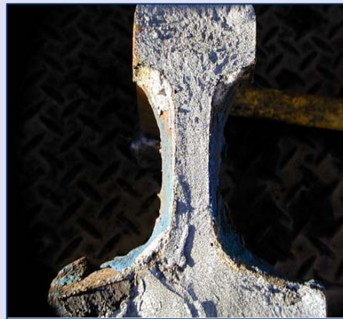
Lack of fusion
